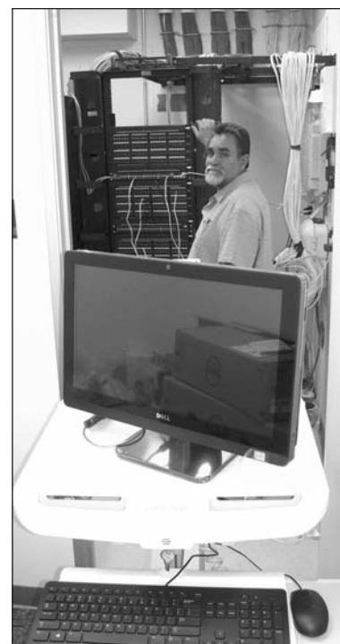
COMPUTER ROOM SET TO HANDLE PATIENTS' NEEDS – Ralph Huerta, facilities supervisor and construction manager for East Valley Community Health Center, shows off the computer room at the new Pomona location which will handle everything from maintaining patients' all-digital medical records to tracking their movement around the facility while they are in for a visit.
