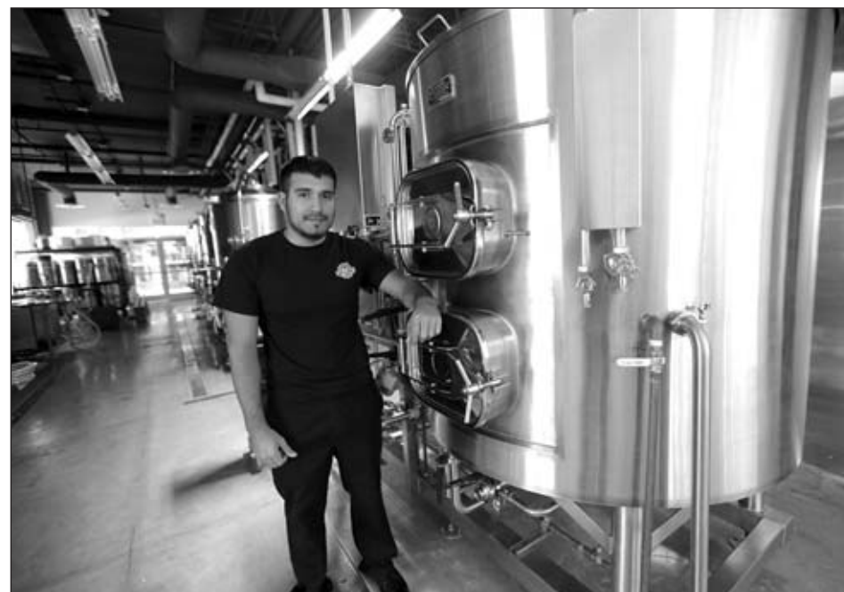
READY FOR BREWING -- Bandelio Delgado, a student "lead" at the new Innovation Brew Works at Cal Poly University Pomona's Innovation Village, shows off the brewing equipment that is ready to go to work making beer.
