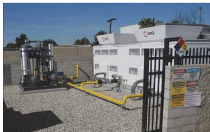
Compressors and storage bottles are an important part of the compressed natural gas fueling facility at the Pomona Valley Transfer Station.
