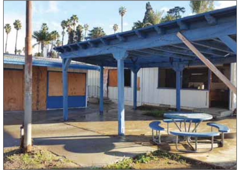
Plans now call for tearing down the original 60-year-old pro shop, at left, and snack shop, at right, at Pomona’s Palm Lake Golf Course and starting over again, possibly using a portable modular building on an interim basis to get the golf course up and running, according to the developer.
