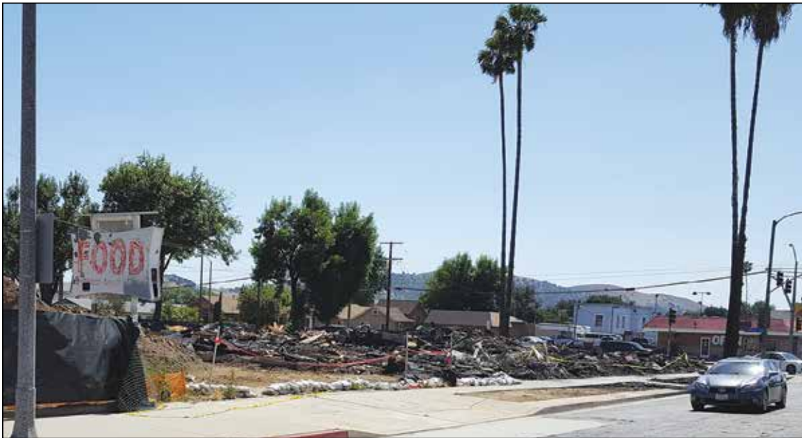
Fire broke out this month at the site of the old Mission Family Restaurant at Mission Boulevard and White Avenue where, as this photo shows, not much is left other than debris and most of the parking lot sign. The structure, a classic diner built in the 1950s, was in the process of being repurposed as a 7-Eleven and other uses.
