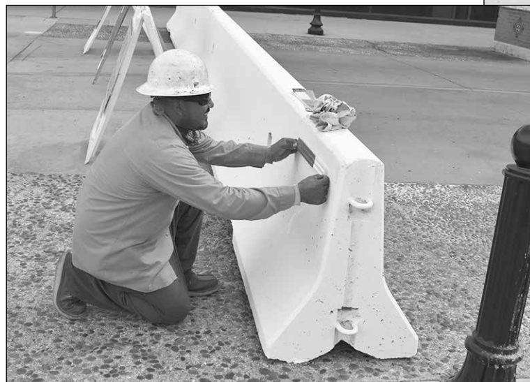
Adam Tapia, of Pomona's Public Works Department, places reflectors and other last-minute touches on the "K-rail" barricades at Garey Avenue and Second Street in Downtown Pomona this month on the first day Second Street was converted to a pedestrian mall with restaurants and other businesses moving things outside on the street.
