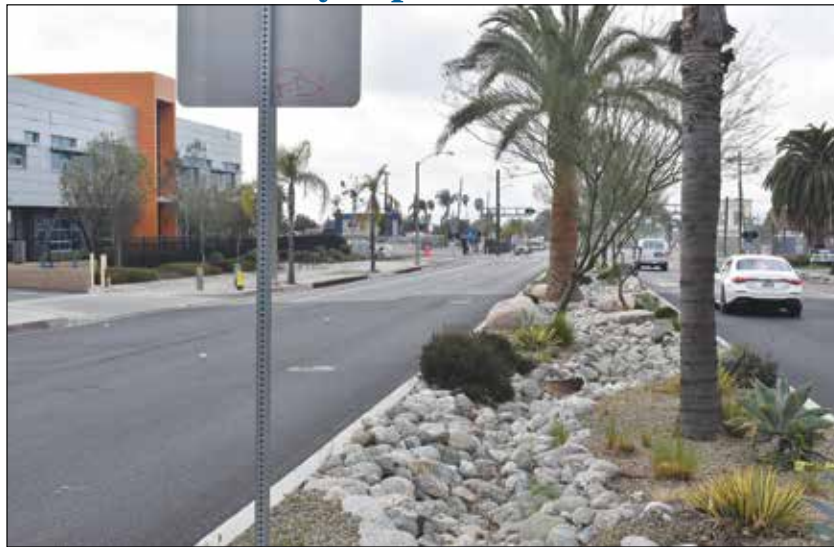
GAREY BOTTLENECKS DOWN TO TWO LANES -- The Foothill Gold Line construction project has reached Garey Avenue where it will narrow down to two lanes and STAY two lanes for the rest of the year. Plus, there will still be a full closure at some point with details not yet being announced. Rush hour delays of up to 15 minutes in both directions just to get through can be expected. Pictured looking southbound on Garey north of the tracks and south of Bonita Avenue is the section of Garey that is becoming one lane in each direction. The photo was taken Monday morning when the work had been expected to begin.
