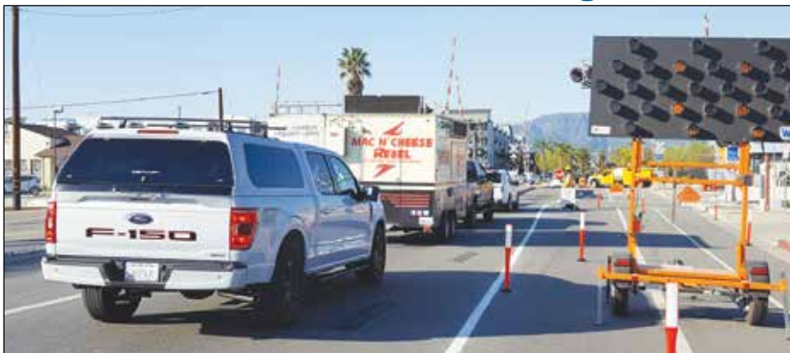
TRAFFIC ON GAREY -- A worker, pictured four cars up at the tracks, holds up a "stop" sign while construction workers move equipment around at rear to do a little digging in the street as they work on relocating underground utilities in preparation for getting the tracks ready at the Garey Avenue crossing for the Gold Line light rail project extension. Also visible is the white line "restriping" that narrows Garey down to one lane in each direction in a project that will continue until the end of the year.
