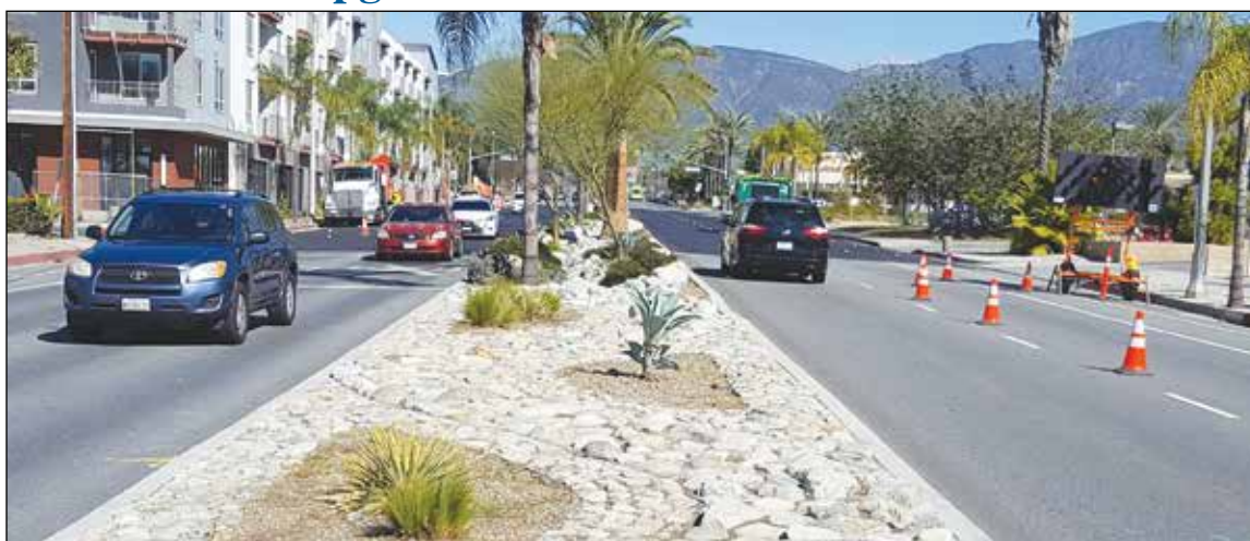
Conventional orange cones were placed down on the first day of lane closures on North Garey Avenue in Pomona late last month. Those cones were quickly replaced with actual lane striping and those little two-inch diameter orange plastic markers that screw into plastic holders cemented to the street. Cars immediately started slowing as they merged into one lane in each direction and made their way through the area of construction.
