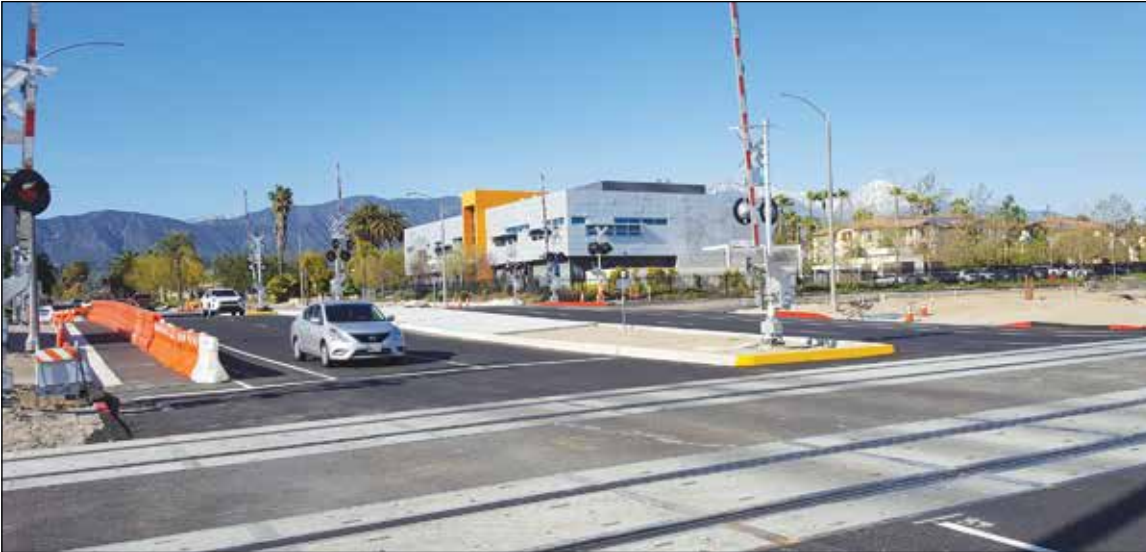
LIVE IN THE AREA? GAREY IS OPEN AGAIN! -- Of course, if you live in the area, you already know the Garey Avenue crossing at the tracks is open again and, as you can see in the photo, it is actually better than before. A full closure of all lanes both north and south on one of the busiest streets in the city went into effect Feb. 1 for what originally was expected to be 45-days because of construction requirements of the Foothill Gold Line line through Pomona to Claremont. The crossing -- and Garey -- was all back in service and open to traffic once again on March 27, or about 10 days late. The Gold Line originates at Union Station in Los Angeles and is expected to bring service to Pomona by 2025.
