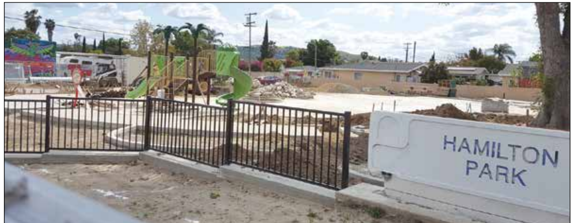
HAMILTON PARK UPGRADES -- Workers are making progress on a $2.7 million upgrade for children of one of the city's oldest barrios. And some of the same people who worked with the city 50 years ago on the park's first development were back to help out this time. Work is expected to be completed by August. (See original story in January 2023 La Nueva Voz at http://www.lanuevavoz.net , click on past issues and scroll down to page 12.)
