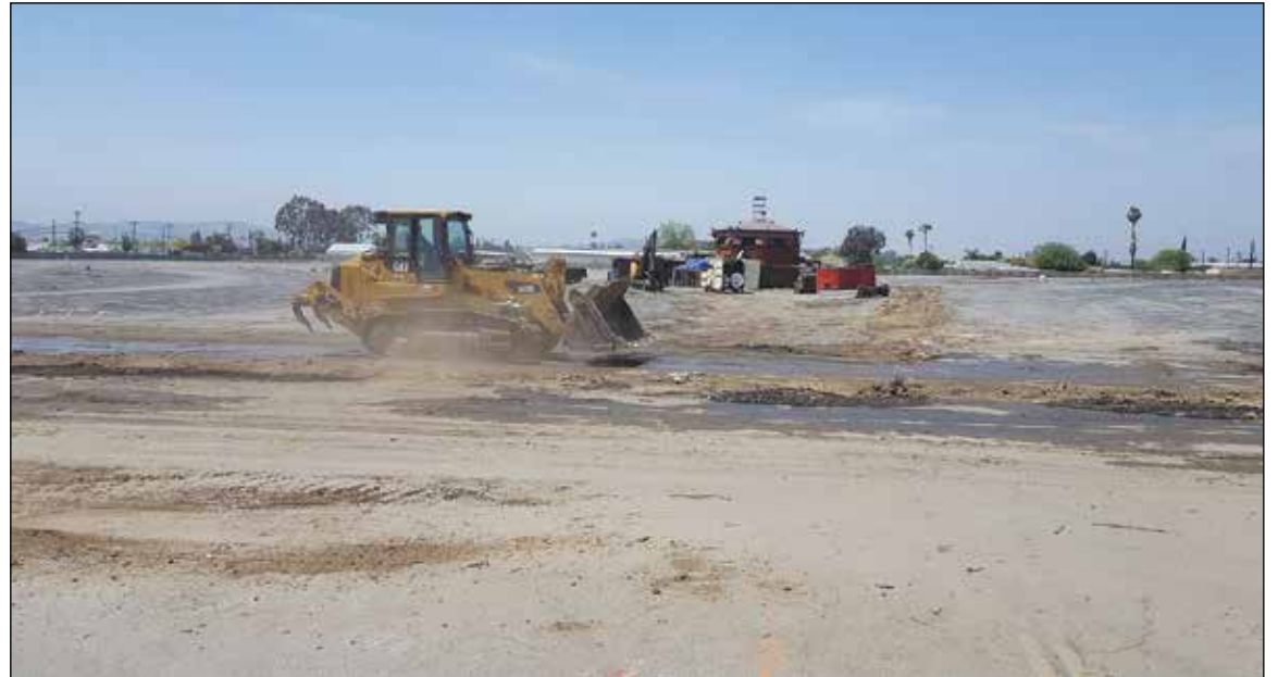
END OF AN ERA -- A bulldozer smooths out the concrete after demolition last month took down four drive-in movie screens, the car window speakers and more, clearing the way for development last month of a 28-acre site which for the past 67 years has been the home of Montclair's Mission Tiki Drive-In Theatre and Swap Meet. As pictured, the projection booth that once housed four projectors, one pointing in each direction to one of the four screens, was still standing but even that was gone the next time La Nueva Voz drove by. Last we looked, the original sign was still standing on the northwest corner of Mission Boulevard and Ramona Avenue. Plans call for building a business park on the site that will include 513,295 square feet of flexible industrial space with new zoning from the present commercial to include both manufacturing and commercial.
